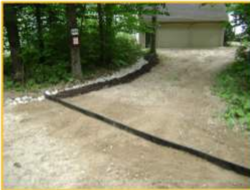
Rubber Razor - strips of hard rubber are partially buried in the driveway, placed on an angle to divert stormwater into an adjacent trench or natural area.
