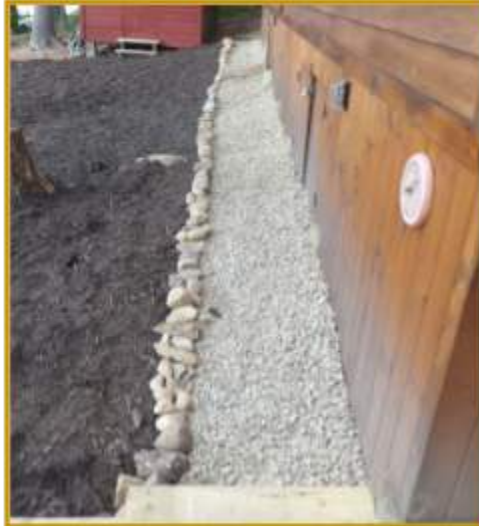
Dripline Trench - Traps roof runoff and directs it into the ground. An alternative to gutters.
