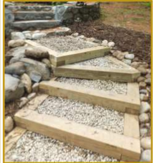
Infiltration Steps - Crushed stone steps that trap stormwater instead of allowing it to flow downhill.
